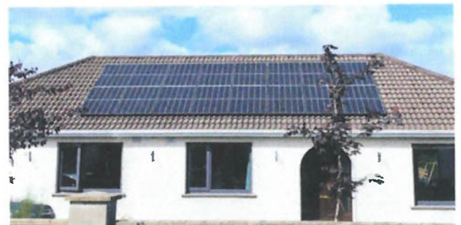
Solar 16 PV panels installed on a domestic home
